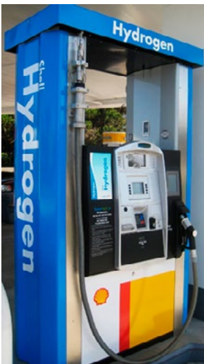
Hydrogen Dispenser at Shell Station. Newport Beach, CA. Source: FuelCellWorks.com
