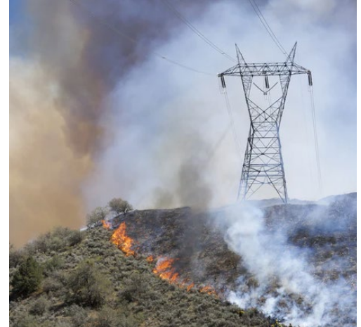
Power line tower in the wildland-urban interface fire area. Photo credit: T&D World
