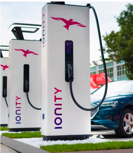
Car charging station
