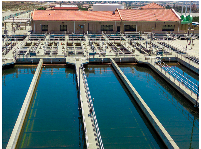
Cucamonga Valley Water District Plant
