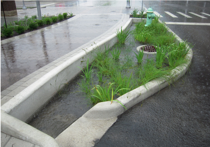
Storm infiltration system in bulbed corner
